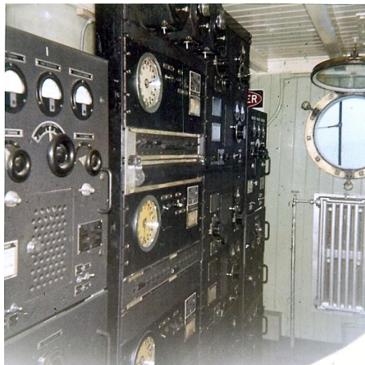
Radio Beacon, located in Radio Beacon Shack as shown above
